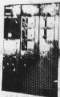
Motor Control Centers
